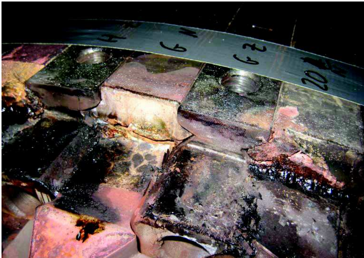
Figure 4: View of NDE rotor shrink seat area after removal of retaining ring
