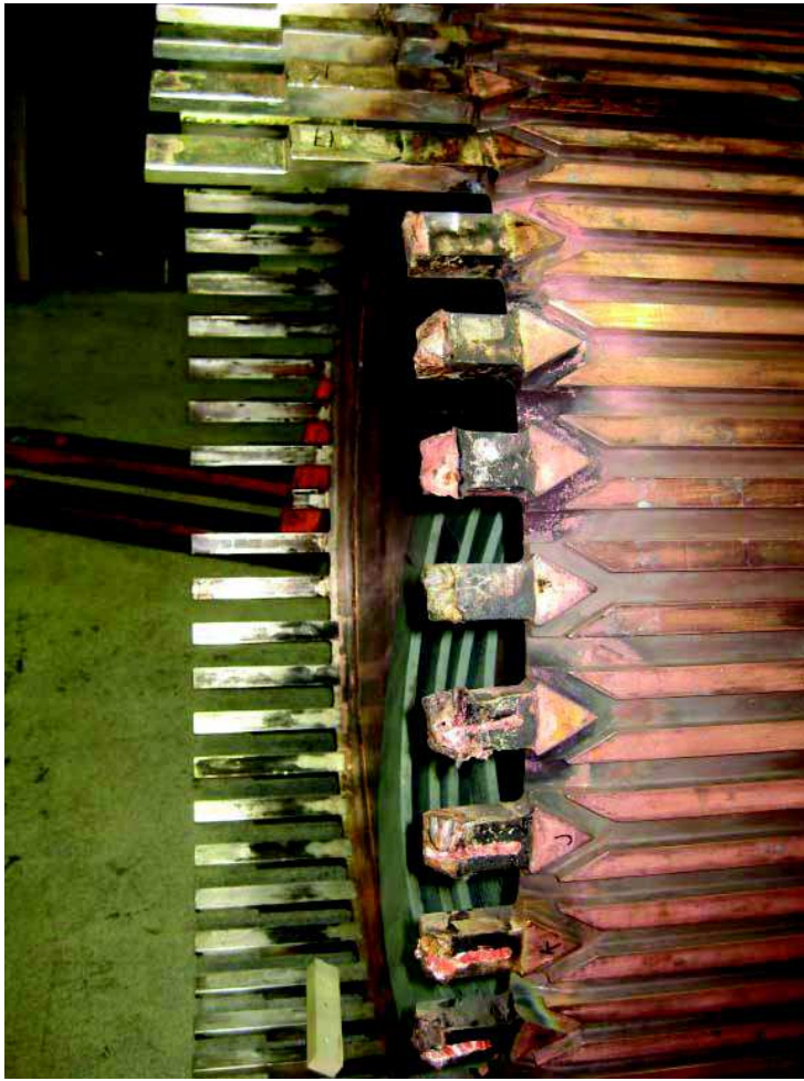
Figure 5: Damper basket NDE, 14 damper fingers were broken off
